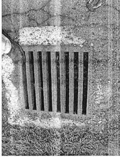
Example- This storm drainage grate at the VA Creeper Trail crossing of South Shady Avenue is an older design and is a safety hazard to bicyclists. It should be replaced as soon as possible.
